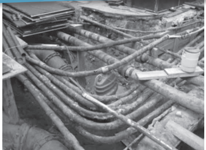
Pipes under Fulton Street in New York City.
